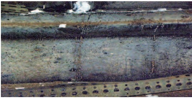
Fig. 4. Visible cracks in prestressed concrete girder
