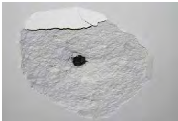
Fig. 3. Detachment of a circular section of ceiling plaster
