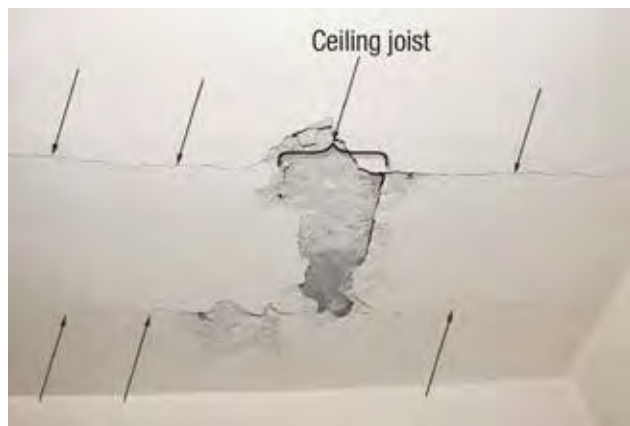
Fig. 2. Cracks perpendicular to the ceiling joist
