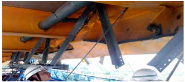
Fig. 4. Main girder deformation after the ship collision with Binh Bridge during CONSON hurricane
