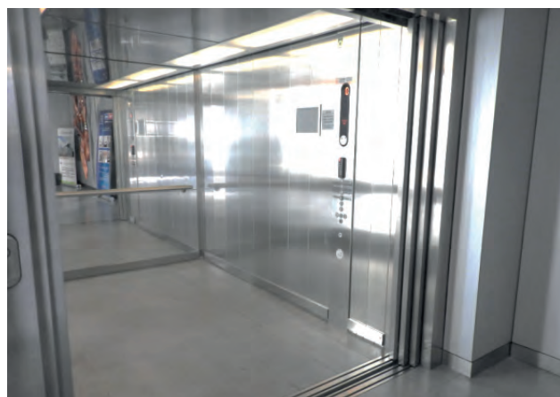
Fig. 28. Elevator in the building
