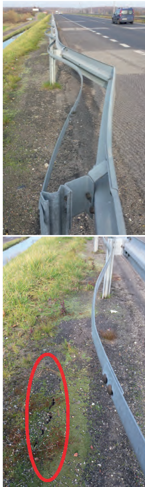
Fig. 16. Longitudinal crack in the crown of the embankment along with the deformed road barrier
