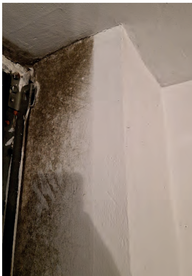
Fig. 3. Biological corrosion visible on the surface of the window reveal
