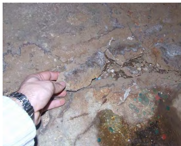
Fig. 3. Detachment of concrete
