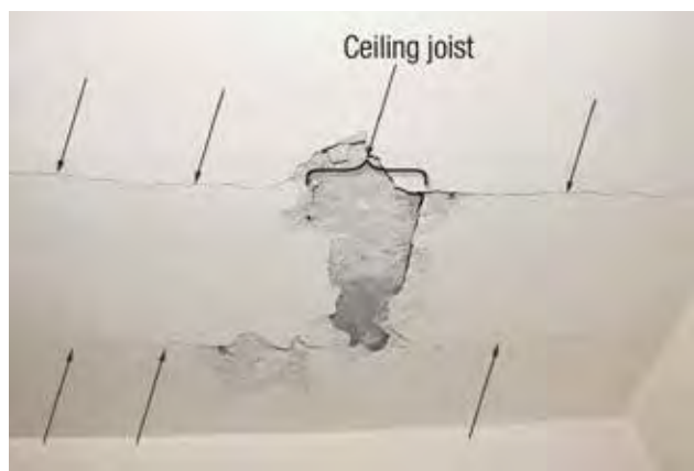
Fig. 2. Cracks perpendicular to the ceiling joist
